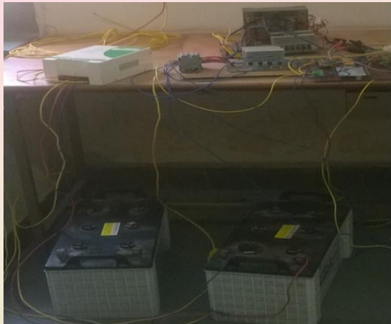
Solar PV Energy Conversion with intelligent Energy Management System
